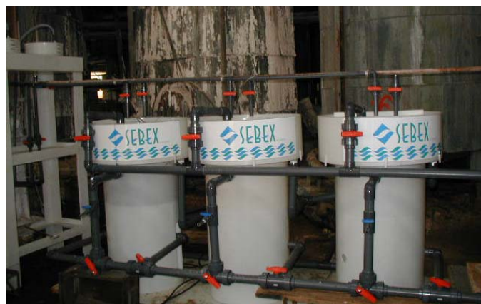
Fig. 3 Connection of experimental equipment for sewage water from blast-furnace circuit treatment (real view)
